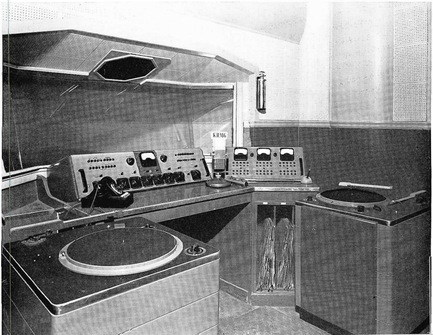
FIG. 5. View of Master Control Room of KRMG, looking into studio B. A Type BCS-1A Master Switching System is located to the right of the 76-C Console. Note location of LC-1A Speaker above the control room window.
